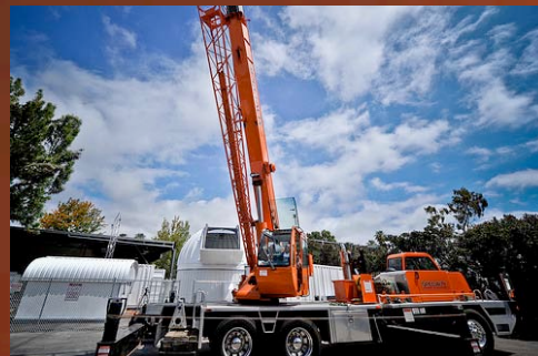
May 2010: Crane to lift a complete, aligned & tested 1m mount, cell and M1 into an 18' Ash Dome. Process takes about 1.5 hours.
